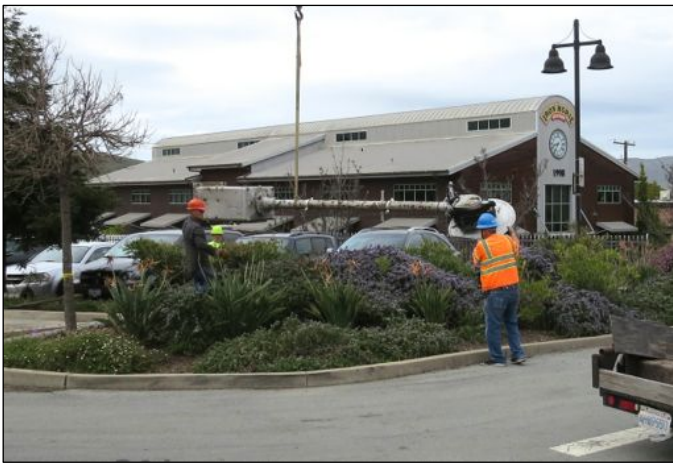
A trackage signal is lowered horizontally to a temporary resting place between parking lot landscaping.
