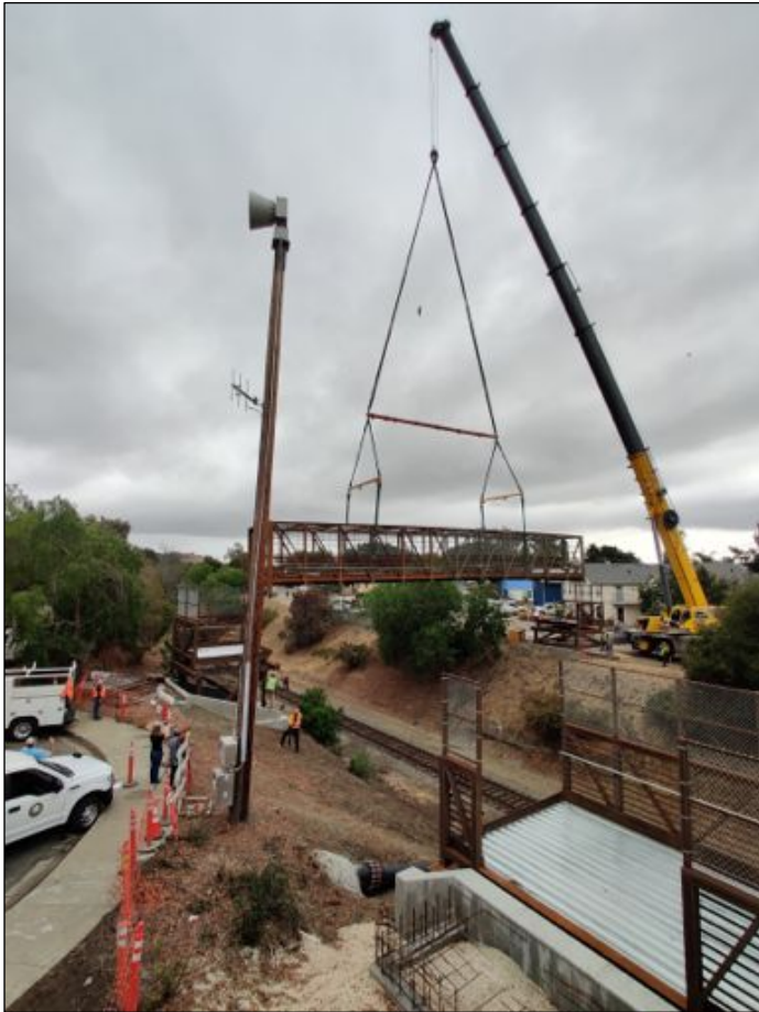
In an operation familiar to the Museum, an extended-boom crane lifts into place the span for a new bicycle and pedestrian bridge over the railroad, north of Mill Street and west of California Boulevard.
