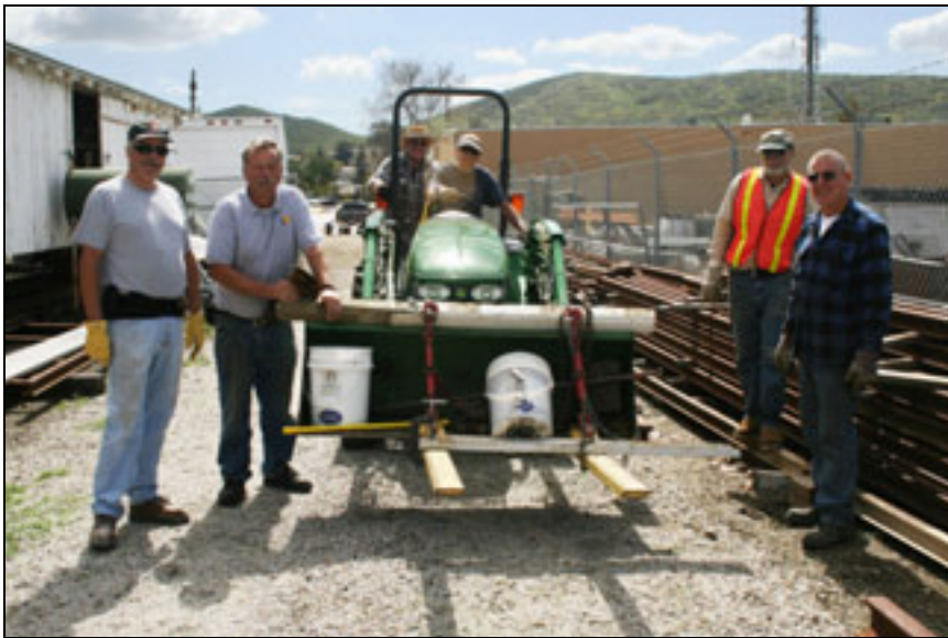
Tom Mitchell, Ted VanKlaveren, Duane Powell, Howard Amborn, Glen Matteson and Tom Cooper get ready for a days' work moving track to the Freighthouse where it will display the boxcars. Photo by Gary See
