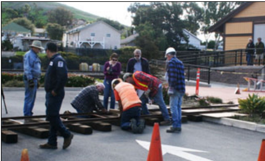
The intrepid crew installs a temporary snap-track across the parking lot in order to unload the boxcars from the truck. Photo by Gary See
