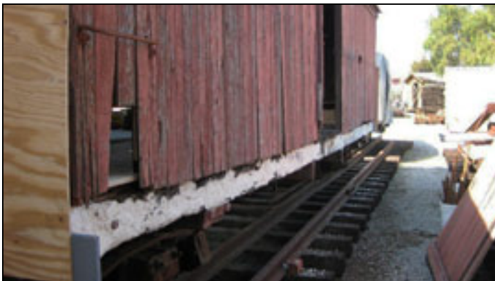
8 The termite damage and rot is not as bad as it looks in the previous picture, and Ted was able to repair the sills and end beams using Liquid Wood epoxy filling material. Photo by Ted VanKlaveren
