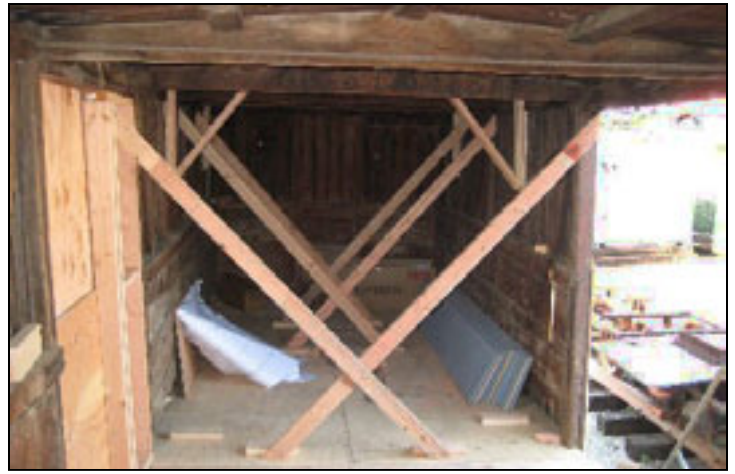
Temporary bracing has been added to stabilize the structure while repairs are conducted. Photo by Ted VanKlaveren
