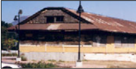
A new foundation was poured under the South end of the building. September 2004 photo by Bill Pyper
