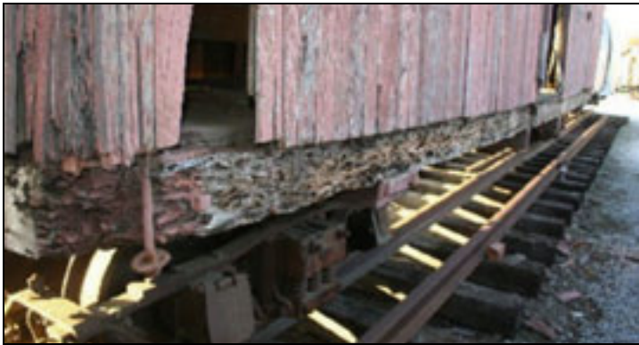
This picture, taken by Ted VanKlaveren, on January 26, 2012 shows the rotted condition of boxcar 706.
